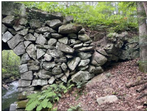
Collapsing southeast spandrel. -photo by Weitzner
