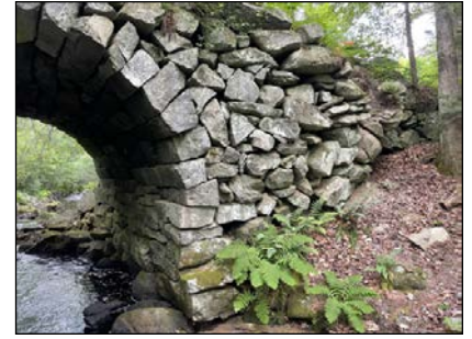
Arch voussoirs on the southeast side of the arch. -photo by Weitzner
