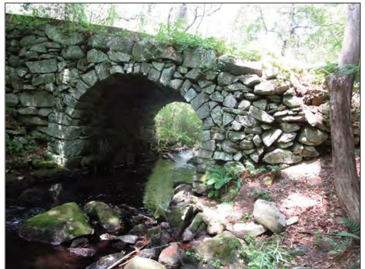
Keystone Bridge June 27, 2021 with right side partially collapsed
