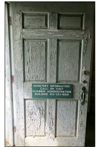
Administration Building Door (note condition)
