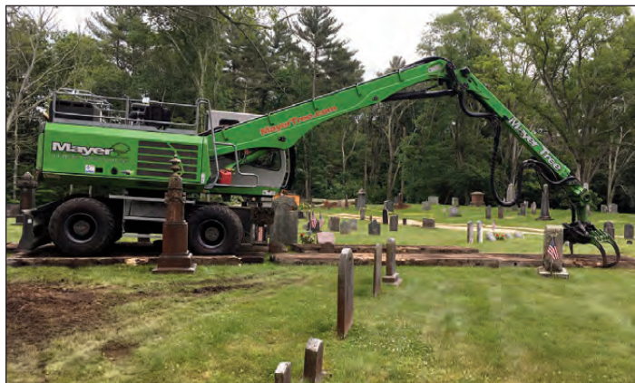
Mayer Tree Service removing trees during June 18–21, 2019. The machine was leapfrogging planks to reduce the impact to the landscape from heavy machinery.
