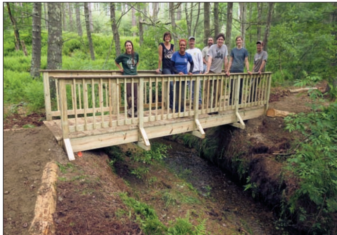
Student Conservation Association crew members and DCR staff stand atop the new bridge along the Swift River trail. From left: Evelyn Cilley, Katie Avery, Jasmine Jones, DCR staff Al Detour and Paul Davis, Ryan Pennesi, Sara Wyatt and Isaac Arndt.
